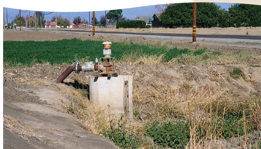
Tail water return pump.
