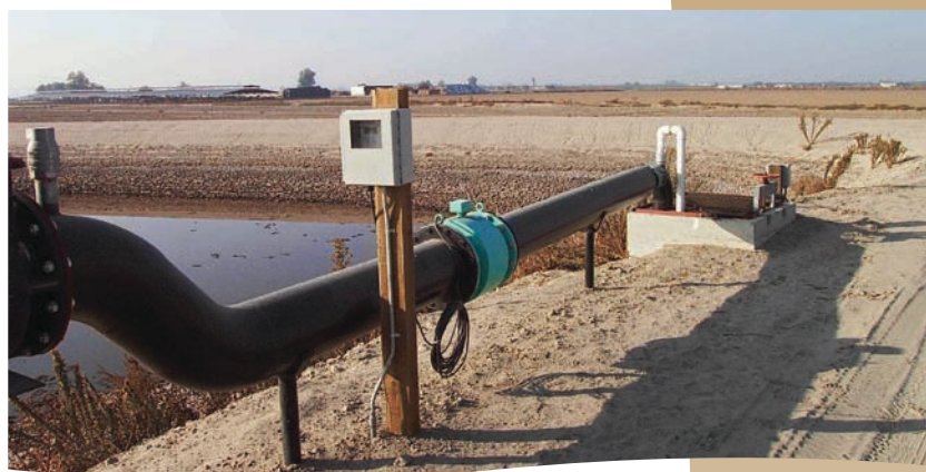
Liquid manure transfer pipeline with electromagnetic flow meter.
