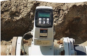
Liquid manure flowmeter.
