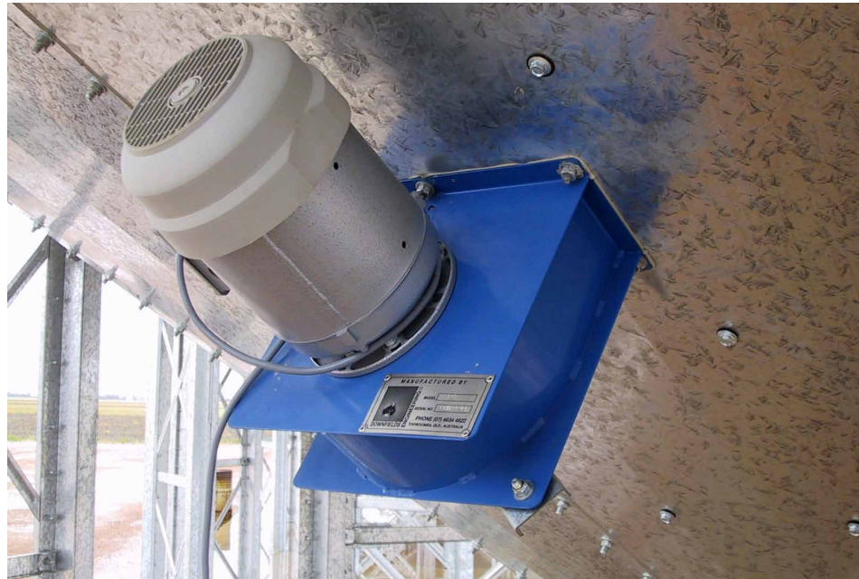
Figure 1: Storage with aeration is important for protecting Australia's markets. (Photo: DAF Qld)
