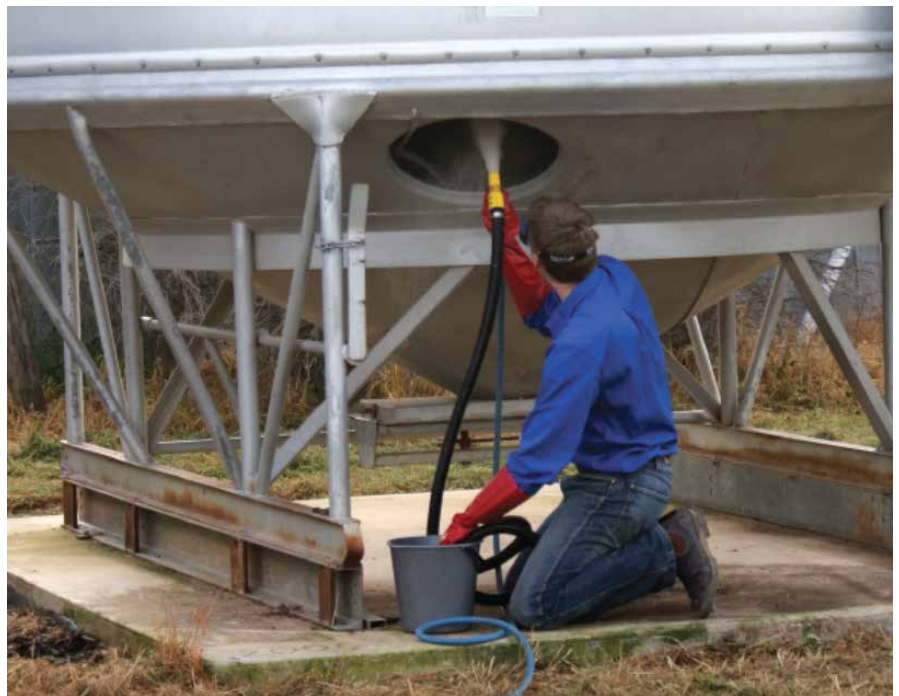
Photo 8: A blower and vacuum gun such as the Venturi gun is the best applicator for inert dusts. Aim for an even coat of diatomaceous earth across the roof, walls and base.
