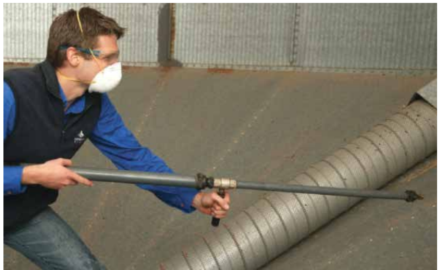
Photo 6: Clean silos, including the silo wall, with air or water to provide a residue-free surface to apply structural treatments.
