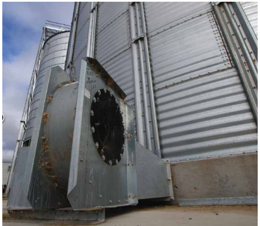
Photo 10: Aeration drying requires careful management, high airflow rates, well designed ducting, exhaust vents and warm, dry weather conditions.
