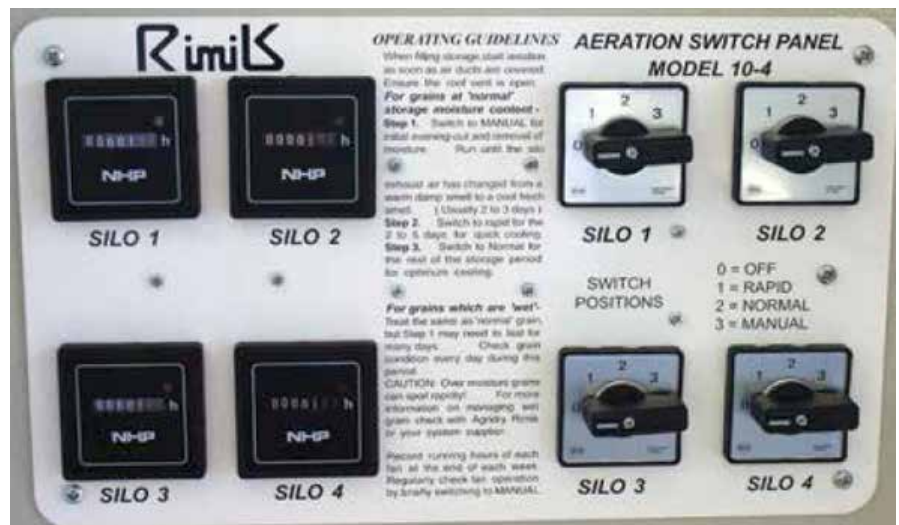
Photo 11: Automatic aeration controllers are the most effective way to cool grain and are designed to manage many storages, from one central control unit.
