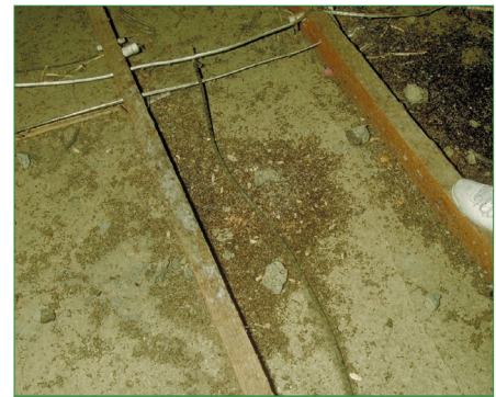
Figure 4. Accumulation of bat fecal pellets on a ceiling.
