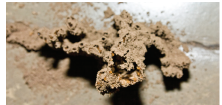
(5D) Swarm tubes emerging from floor crack.
