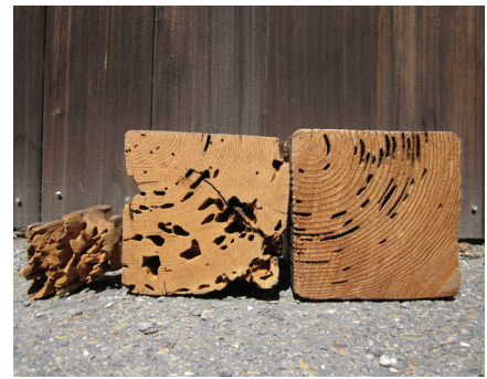
Figure 2. Damage to wood by dampwood (left), drywood (center), and subterranean (right) termites. (R.L. Tabuchi, U.C. Berkeley)
